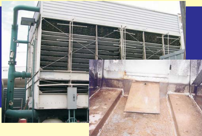
Tower basin in poor condition
